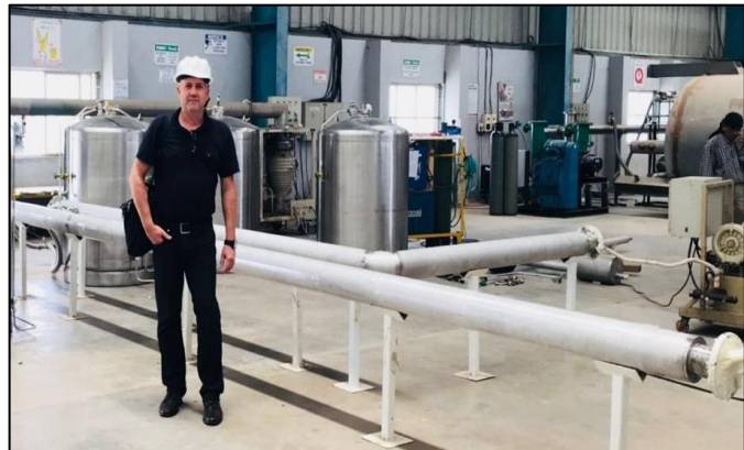
Vacuum Insulated LNG transfer cryogenic pipeline
